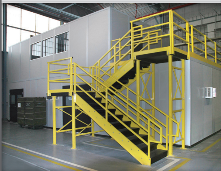
Second story in-plant office, over in-plant shop; utilizing InPlant's 3" Heavy-duty Steel System & FRP Wall Panels.
