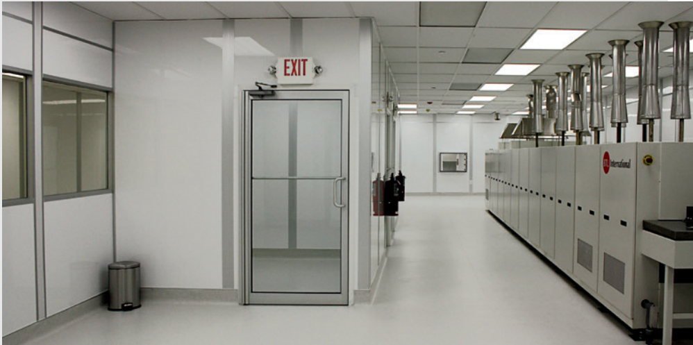
Temperature controlled & dust-free white room
