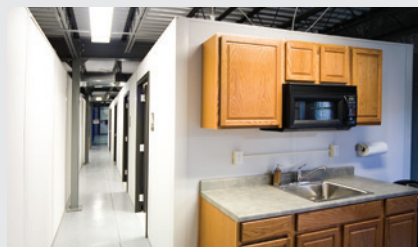
Vinyl Faced Wall Panels partitioning administrative offices
