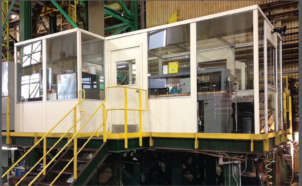
Protected controlling equipment with full glass for supervisory vision
