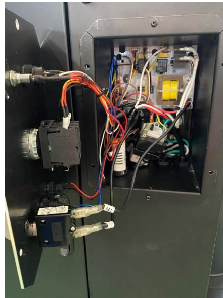
Figure 8: Control Panel/Box Wiring
