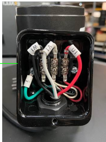
Figure 16: 110V Wiring, Junction Box
